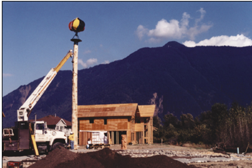
Photo of a wind turbine being set up in the centre of the spiritual healing garden
